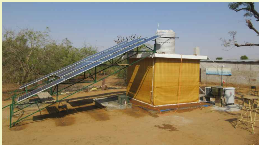
Pusa-Farm SunFridge - a gridless, batteryless cold store running successfully in village Picholiya, Ajmer, Rajasthan
