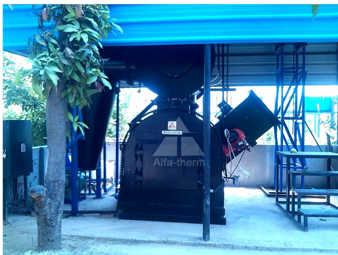
Fig. 1. Incinerator facility at IARI, New Delhi
